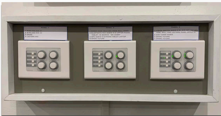
EASE OF USE YAMAHA DCP WALL CONTROL PANELS: LOCATION HALL
